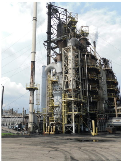
Calgon Carbon Corporation's Pearl River Plant, Bay St. Louis, Mississippi
